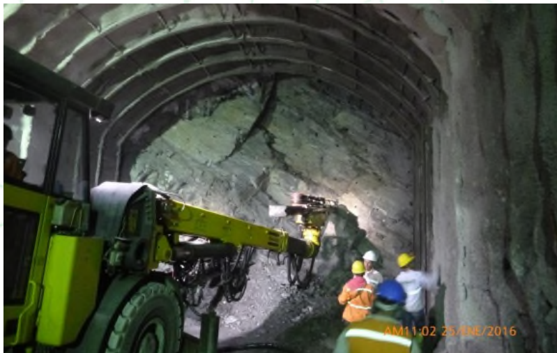
Final Phase of the excavation of a tunnel on the replacement roads of Ituango Hydroelectric Project. Taken From > http://www.elcolombiano.com >
